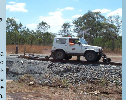
A hi-rail vehicle towing the trolley with GPR antennae. The data logging system is located within the vehicle allowing for safe and efficient operation.
