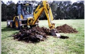
TYPICAL WASTE MATERIAL FOUND BURIED BENEATH SITE
