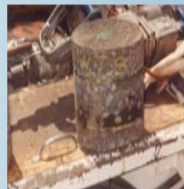
Core taken at location referenced from radar data showing clear delamination between asphalt layers.
